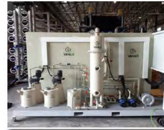
Continuous Stirring Tank Reactor (CSTR)
