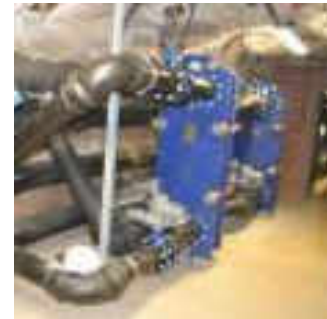
Mine water plant Reiche Zeche
