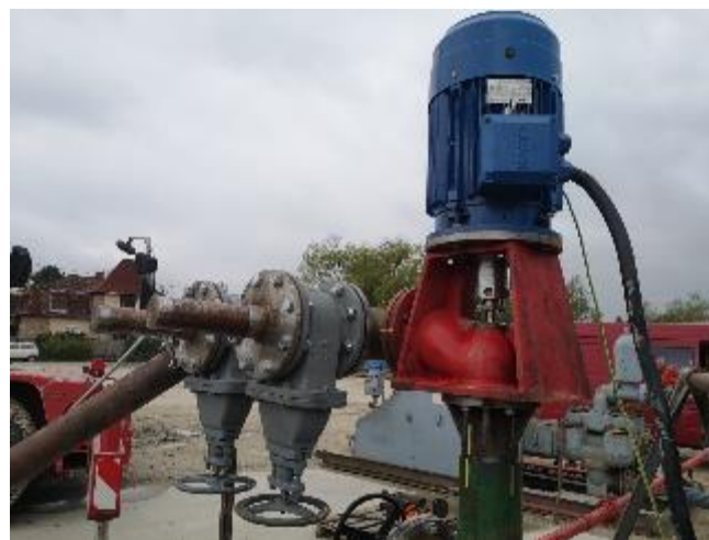
Wellhead during welltest
