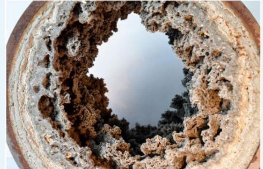
Cross sectional view of a geothermal reinjection pipe showing heavy silica scaling.
